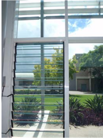
Figure 16: Solar gain through northern aspect glazing (taken at 12:44pm on 7 th March)
