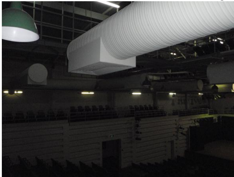
Figure 20: Concert Hall HVAC diffusers
